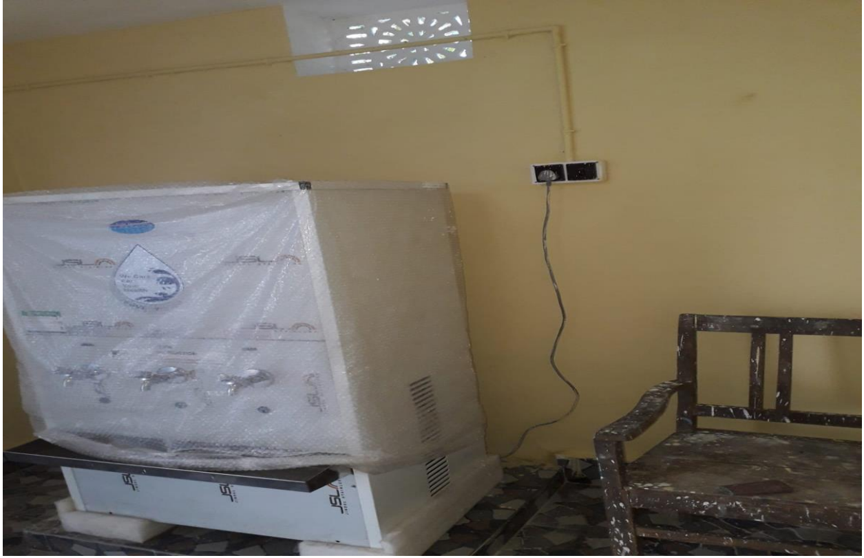
New Aquaguard Machine with Cooler
