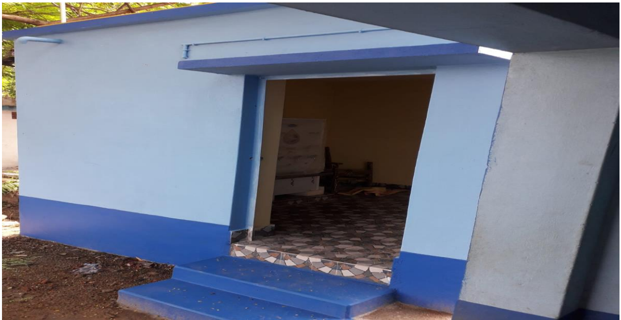
New room for Aquaguard Machine
